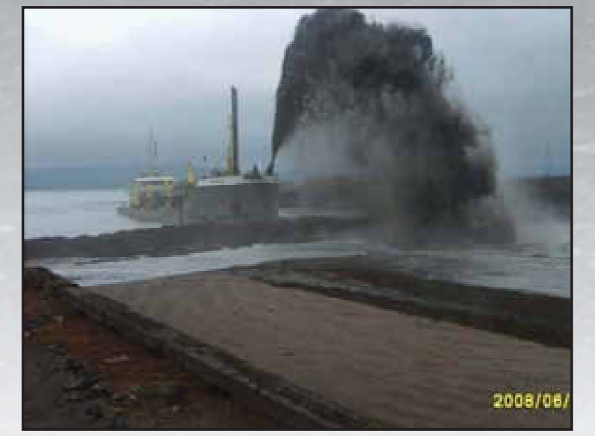
Infilling of the basin with dredged sand using "rain-bowing" method with the southern section of the basin now shown to be partly infilled
